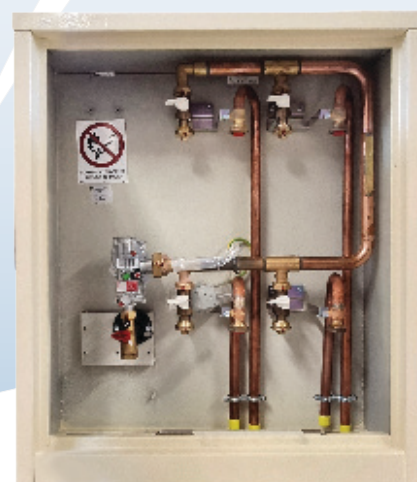
Outdoor gas technical enclosure
